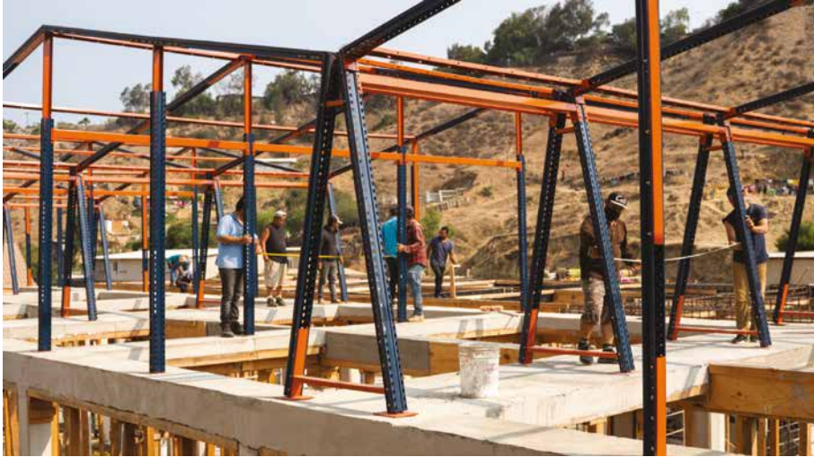
Figure 4. Here, a team of migrant residents skilled in welding and construction install the blue and orange Mecalux metal frames as roofing systems on Santuario Frontera. Photo: UC San Diego Center on Global Justice.
